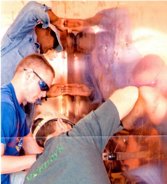
Volunteers from Topeka Bible Church and Grace Bible Church work on the copper.
